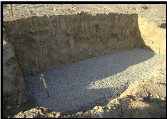
The hole should be excavated prior to delivery and to the appropriate elevation. The system is to be installed on 6" of level rock backfill.
