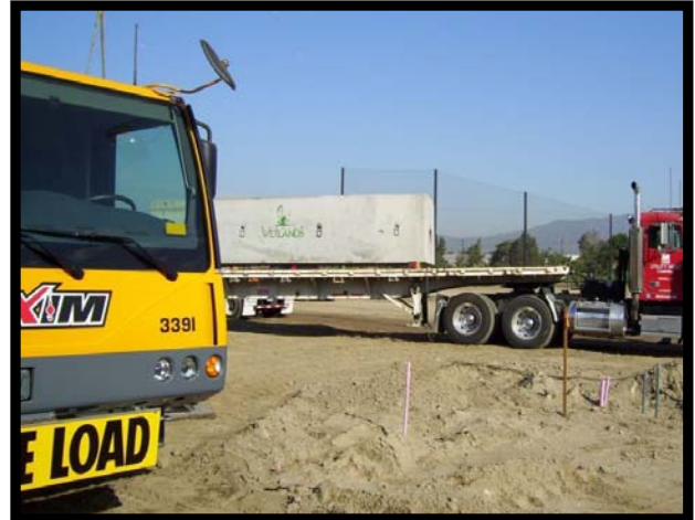
Delivery truck is positioned to off Load Modular Wetland with the crane standing by (contractor to provide the crane).
