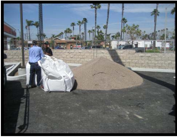
The delivered wetland media is to be prepared to be washed and mixed by the contractor.
