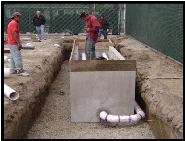
Appropriate size outlet pipe is connected into the Modular Wetland discharge chamber and appropriately routed.
