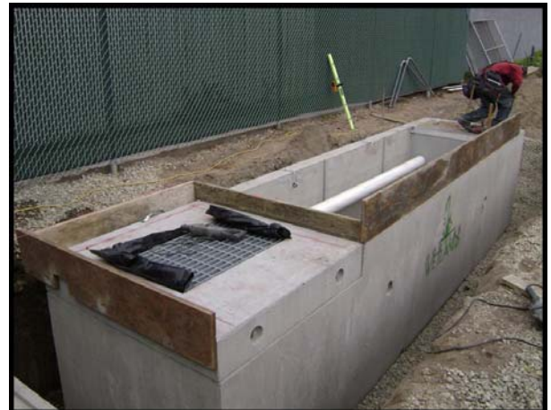
The curb and gutter form is built in the appropriate configuration along the outer perimeter of the Modular Wetland.
