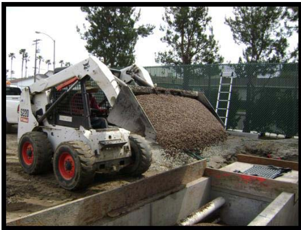
Approximately 8.5 cubic yards of wetland media is carefully placed in to the Modular Wetland.
