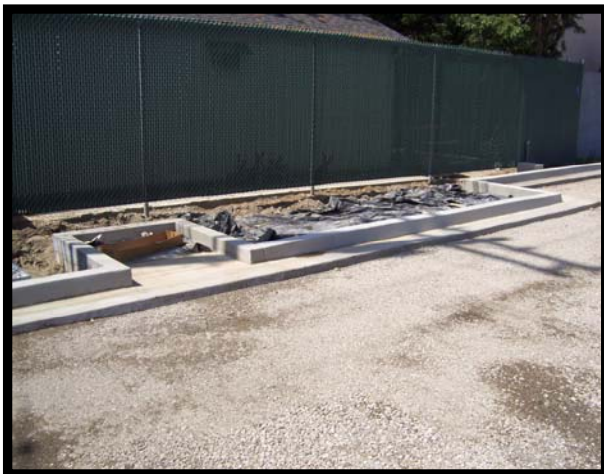
The curb and gutter are pored and the site is ready for pavement.
