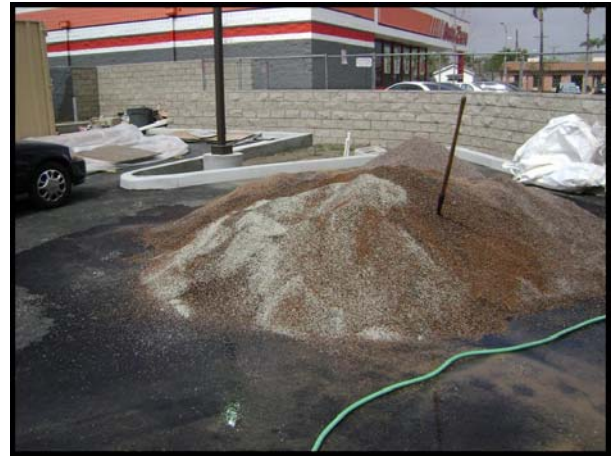
The wetland media, mixed per manufactures recommendations, is now ready for installation.
