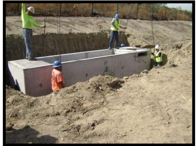
The Modular Wetland Is set into place and the lifting knuckles are detached. Elevation should be confirmed.
