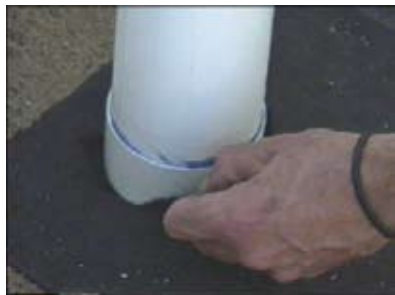
Slide the pipe through the geotextile and the hole made in the Atlantis module.
